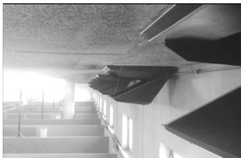
• Air inlets in ceiling
